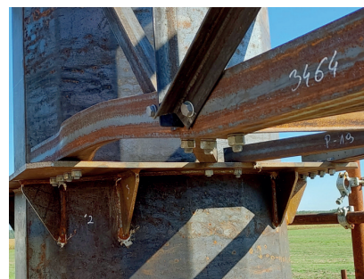
Photo 6. Deformation scheme of the truss type socket of tension pole (III-GM-4)
