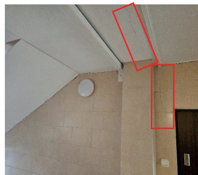
Photo 5. New cracks on the ground floor near apartment no. 9, as of November 2025
