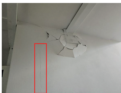
Photo 4. A square pipe element of the tie rod structure on the third floor has been torn out and a new crack has appeared on the wall, as of August 2025
