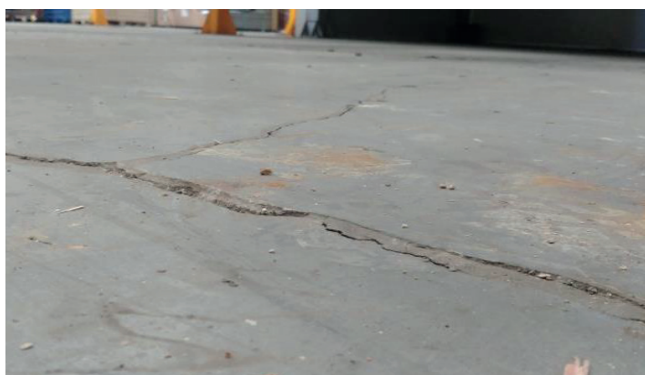
Photo 3. An example of vertical displacement showing floor cracks around technological equipment
