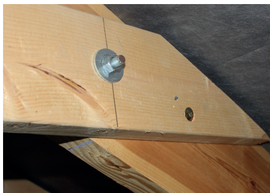
Photo 4. Example of using incorrect connectors
