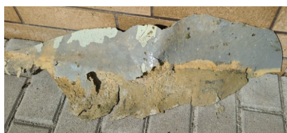
Photo 7. Clear separation of the polyurea from the concrete surface, separation of the primer from the concrete base, and separation of the polyurea from the primer
