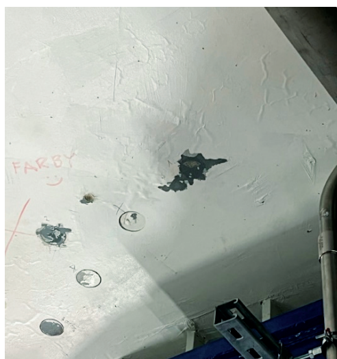
Photo 11. Concrete surface covered with osmotic-diffusion bubbles
