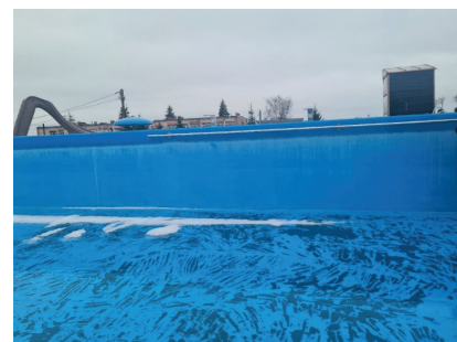
Photo 10. Damaged UV protective layer on an outdoor swimming pool
