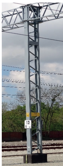
Photo 1. The intermediate pole of a railway catenary gate
