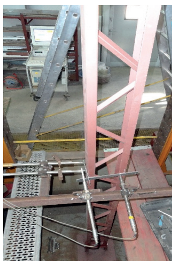
Photo 2. The pole failure due to loss of stability flexural-torsional buckling – general view
