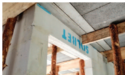
Photo 1. Incorrectly assembled lintel [4]
