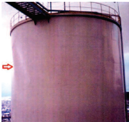
Photo 5. View of deformed silo shell
