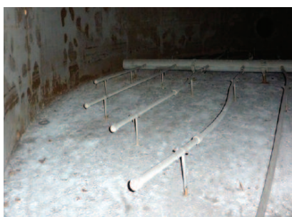
Photo 1. View of a section of the bottom of the steel tank Fot. 1. Widok fragmentu dna stalowego zbiornika
