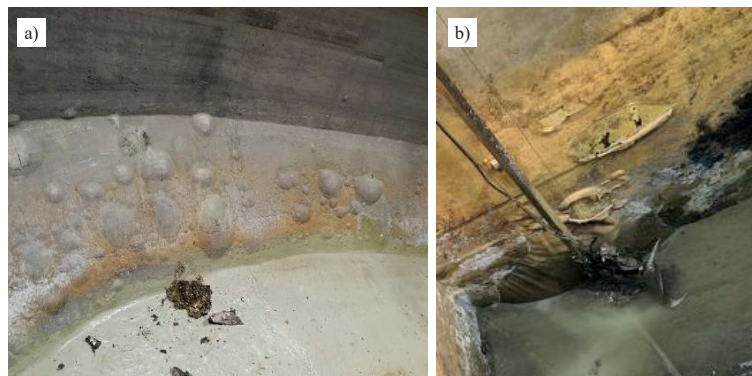
Photo 2. Osmotic activity sector – the substrate initiating the blistering process (a) [8]; osmotic bubbles at the junction of the wall with the bottom and steel elements in a tank in a sewage treatment plant (b) [8]
