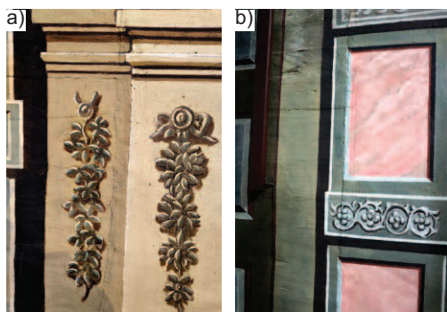
Photo 2. Connection of the polychromes on the canvas and polychromes painted directly on the wood: a) on the right wall of the left transept [photo: K. Matyszewska-Fuszara]; b) on the left wall of the right transept
