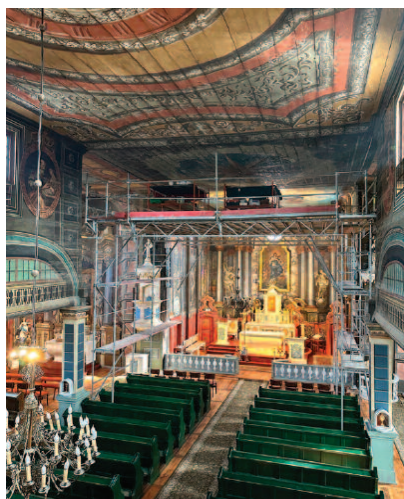
Photo 5. View of the church interior and the polychrome entitled Marian Star on the ceiling at the intersection of the main nave and the transept – during renovation, March 2024 Photo: K. Woszczenko
