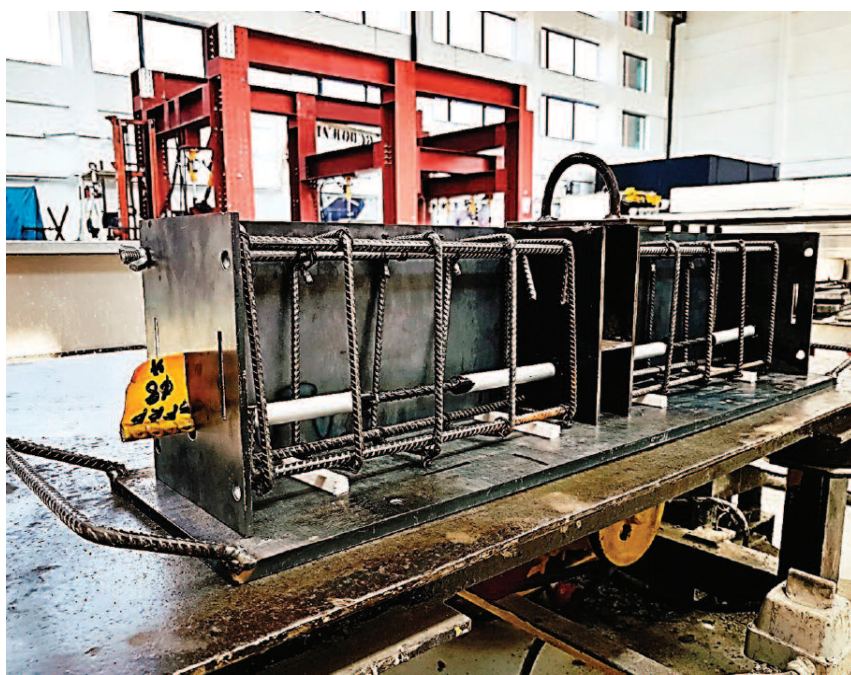
Sample reinforcement during assembly in the mol. Only the central composite bar is routed through the mold walls. The other holes are mounting holes for screws
