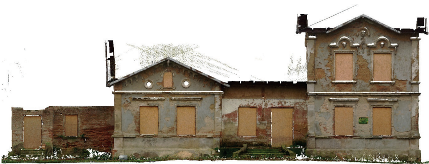
Photo 2. View with RGB information of the front elevation of the manor house in Kliczewo Małe
