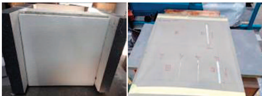
Ściana testowa z defektami systemu ETICS Test wall with ETICS defects
