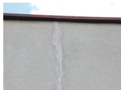
Fot. 4. Spękania na attyce Photo 4. Cracks on the attic
