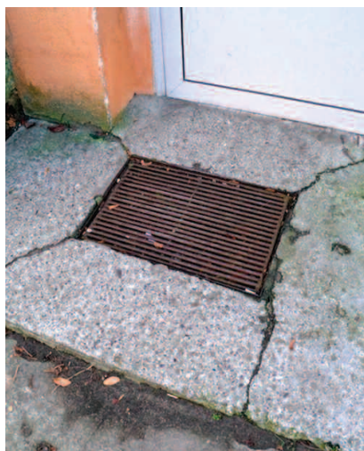
Fot. 3. Zniszczony podest wejścia do budynku Photo 3. Destroyed landing of the entrance of the building
